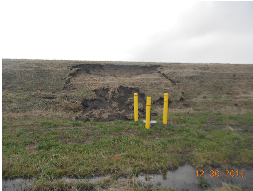
Figure G.1. Photo of 2015 sloughing prior to repairs.
