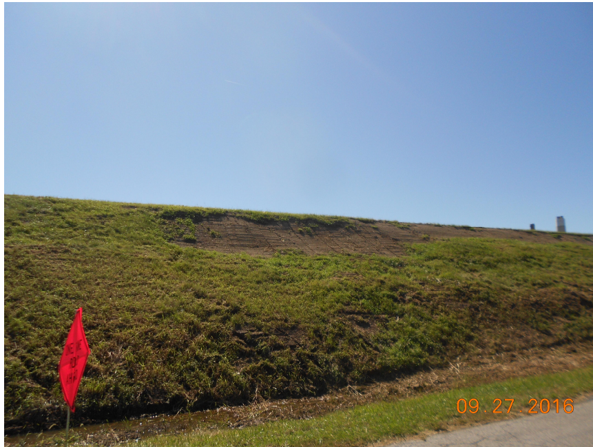
Figure G.3. Photo of 2015 sloughing area after repairs.
